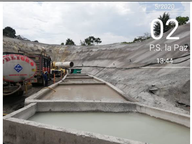
Wastewater treatment units in La Paz exit portal UF6
