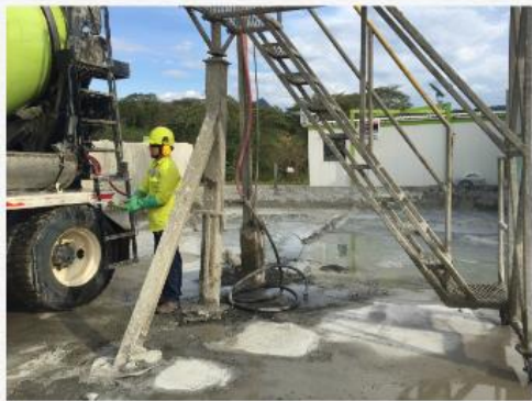
Water treatment capacity in the Argos Cement plant located in Cartama UF 4
