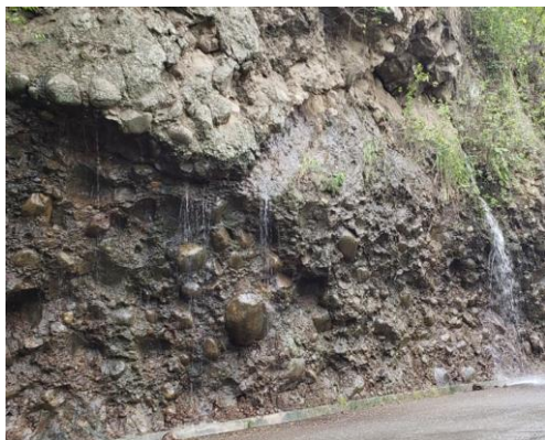
Water springs in UF 2 K 33+100 to K33+760
