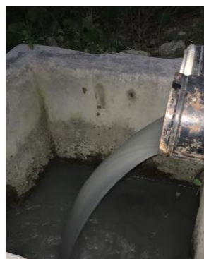
Color and Turbidity in wastewater discharge (tunnel UF3)
