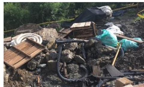
Inadequate storage of wastes and excavation material
