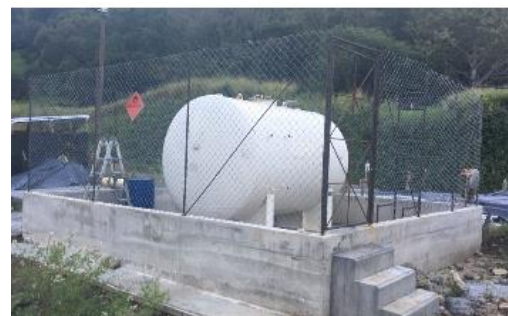
Adequate control spill infrastructures
