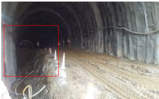
Figure 3 Risk of falling at the entrance of Tesalia Tunnel. Lack of signalling and protection barrier.
