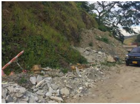
Figure 7. Debris and excavation material in different places than the authorized.
