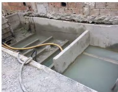
Figure 11. WWTP without protection barrier in flocculant section in Tesalia exit portal.
