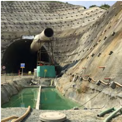
Figure 19. Air control and WWTP in Tesalia exit portal.
