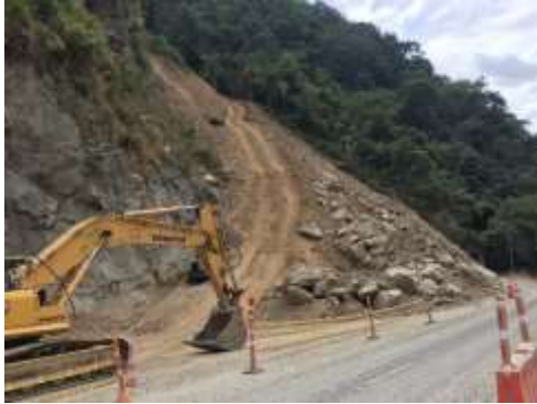
Figure 1 Landslide at the entrance portal of Irra Tunnel
