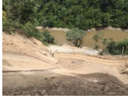
Figure 2 Landslide at the entrance portal of Irra Tunnel from the top.
