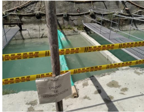
UF 2. Tesalia Tunnel Water Treatment
